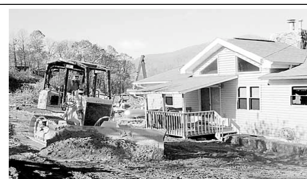
Figure 18. A bulldozer removes soil from a yard at Barber Orchard in Haywood County, North Carolina in 1999 (Raleigh News & Observer)
